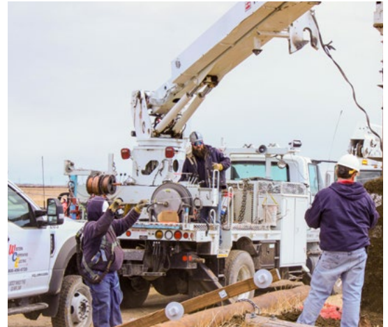
From left: Ellsworth Line Crew members Dustin Wacker, Tyler Renard and Line Foreman Mark Klein at work.
