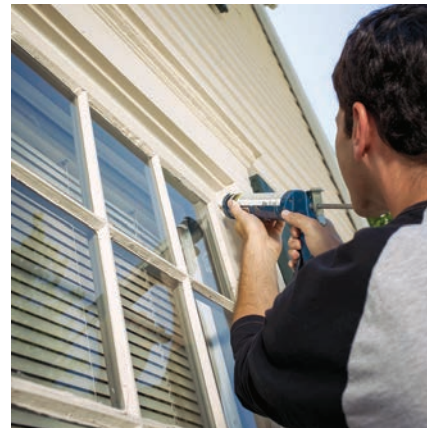
Sealing air leaks in your home can help you save 10% to 20% on heating and cooling bills. Apply caulk around windows, doors, electrical wiring and plumbing to seal in conditioned air.
