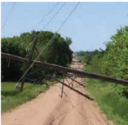
Just two weeks after the winter storm, a tornado caused outages to 900 meters.
