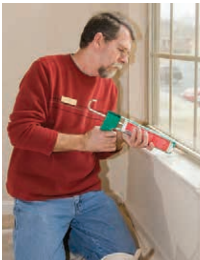
Avoid heat loss by adding weather stripping and caulking to your windows.
